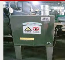
Direct gas heating system
