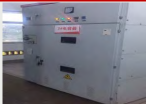
Using electrical power compensation device
